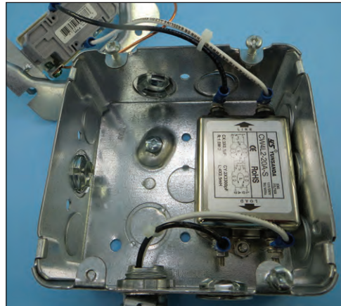
Figure 6: AC Line Filter mounted in an AC outlet box.
